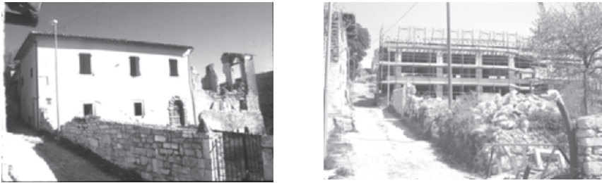
Figure 3. The building repaired in the 80s and partially failed, has been demolished and an r.c. structure rebuilt.
