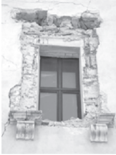
Figure 11. Poor results of applied injection.
