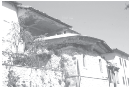
Figure 7. Roof hammering the masonry walls.
