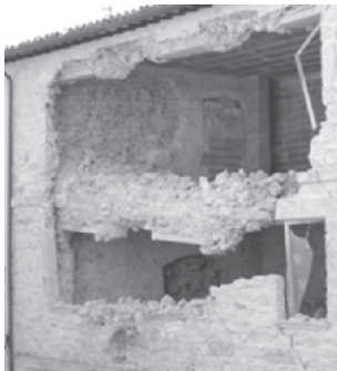
Figure 6. Out-of-plane collapse of a wall with r.c. tie beams.
