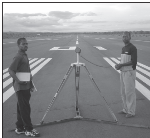
Figure 115. The beginning of runway 01 at Tete Airport (Mozambique). The number 01 is painted in enormous digits so that a pilot can clearly read it during his landing procedure. The painted number equals the magnetic azimuth of the runway in units of 10 degrees, i.e. the magnetic azimuth of this runway is 10^\circ .
