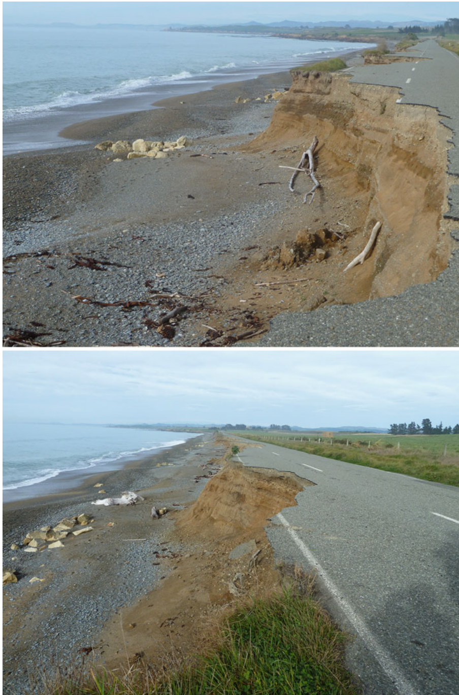
Coastal Erosion, Figure 1 Coastal erosion occurring on the North Otago coast of South Island, New Zealand. The management strategy has been to abandon the road after attempts to build protective rip-rap structures failed (source of debris on the beach) (Photo: Wayne Stephenson).
