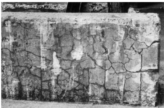
Fig. 9.3 Concrete cracking due to ASR
