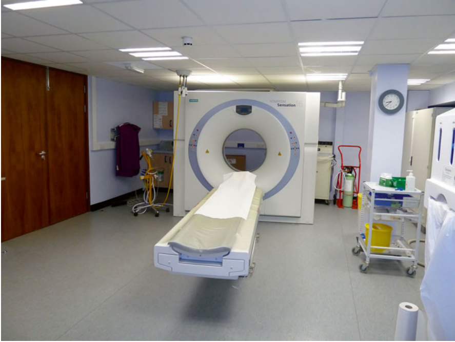
Fig. 9.1 A well configured imaging room allowing plenty of space for patient bed, equipment and staff to the side of the imaging table
