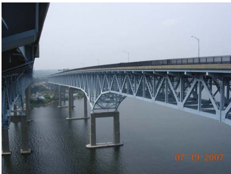
Fig. 7.8 Goldstar Bridge over the Thames River in New London, Connecticut. Multiple solar-powered nodes monitor strains and vibrations at key locations on this structure
