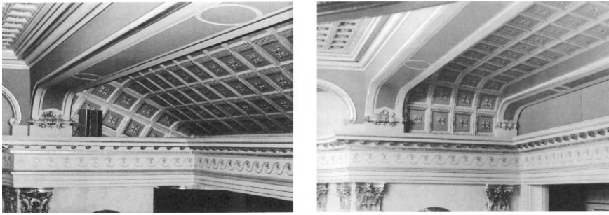
Fig. 6.20 Ceiling above the orchestra in the Staatsoper Berlin (after Marx and Tennhardt, 1991)
