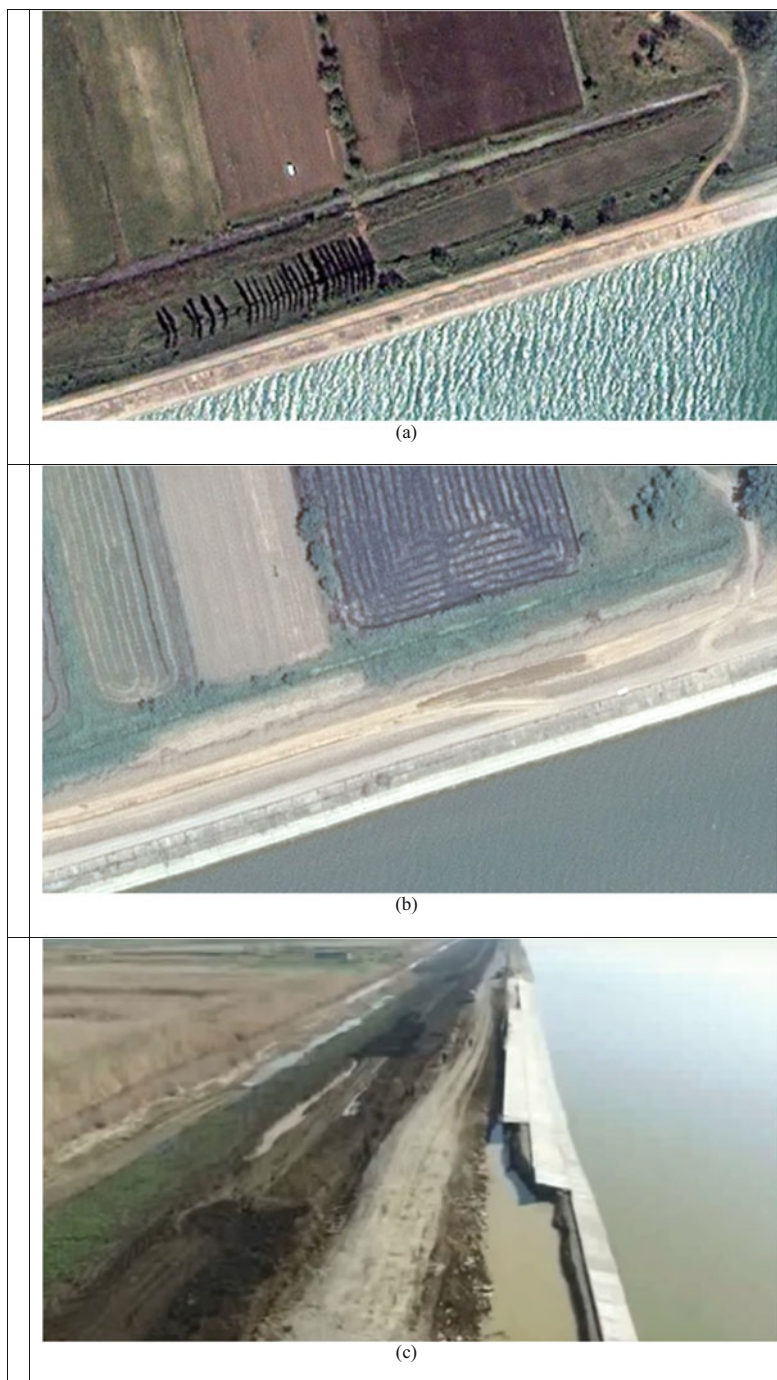
Fig. 11 Section of the northern dam of the Kryukovskoye Reservoir: (a) before its damage on 3 March 2013, (b) after work to strengthen it on 2 August 2014, (c) the damaged section, 1 April 2017
