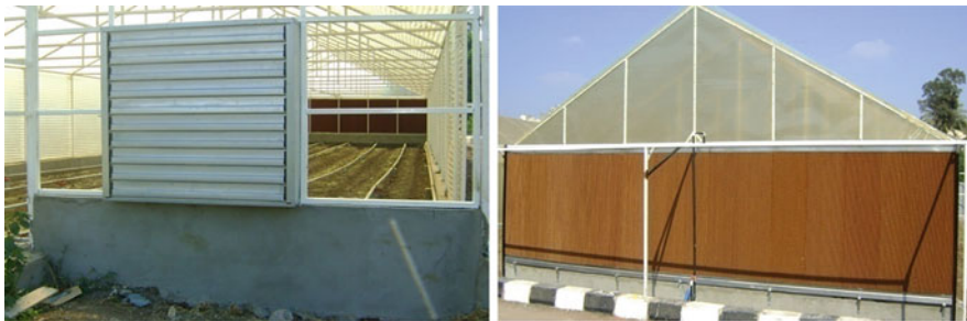
Fig. 16 Fan and pad cooling system. ( Left ) Exhaust fan located on the leeward side of the greenhouse, ( right ) cross fluted cellulose pads placed vertically in the opposite wall of exhaust fans
