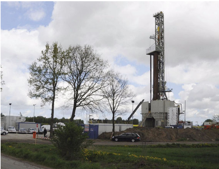
Fig. 2 Shale gas rig in Lebien, in northern Poland, where Lane Energy Poland company does test drilling ( http://www.mlive.com/business/mid-michigan/index.ssf/2011/06/is_growing_shale_gas_revolutio.html )
