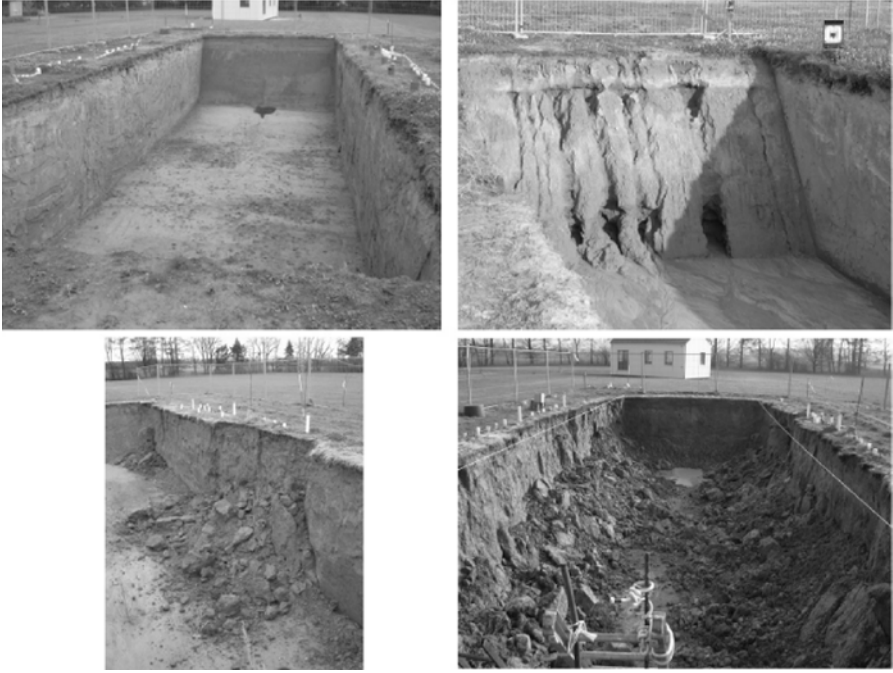
Fig. 8. Upper left: June 2004 – after excavation of the test trench; Upper right: first localised failures (January 2005); Lower left: eroded inclined sides; Lower right: generalized failures (February 2005)
