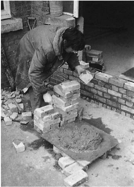
Fig. 3. A bricklayer's apprentice encountering the irritant and allergic risks from cement
