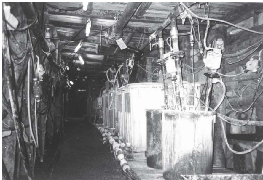
Fig. 4. View of the grout plant used for field tests and first full scale application.
