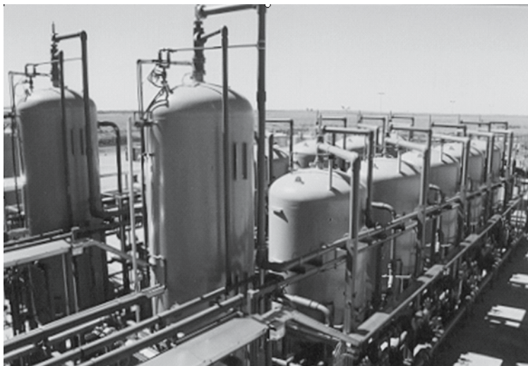
Fig.7. View of the U processing plant showing part of the IX columns for U capture.
