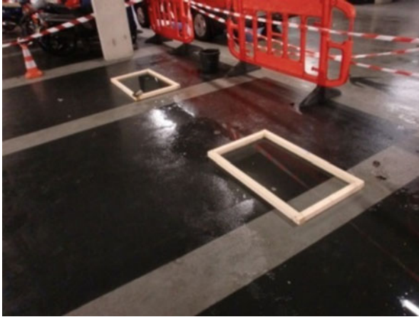
Fig. 26 Second leakage test on crack AB
