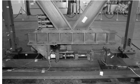
(b) The MR damper and its supporting brace.
