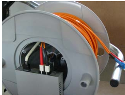
Fig. 4. A close-up of the cable deployment system
