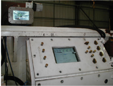
Fig. 7. The flameproof enclosure housing the operator display, input controls and computing hardware.
