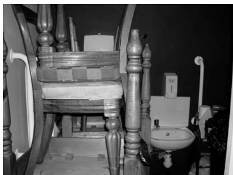
Figure 23.4. Accessible toilet used as storage
