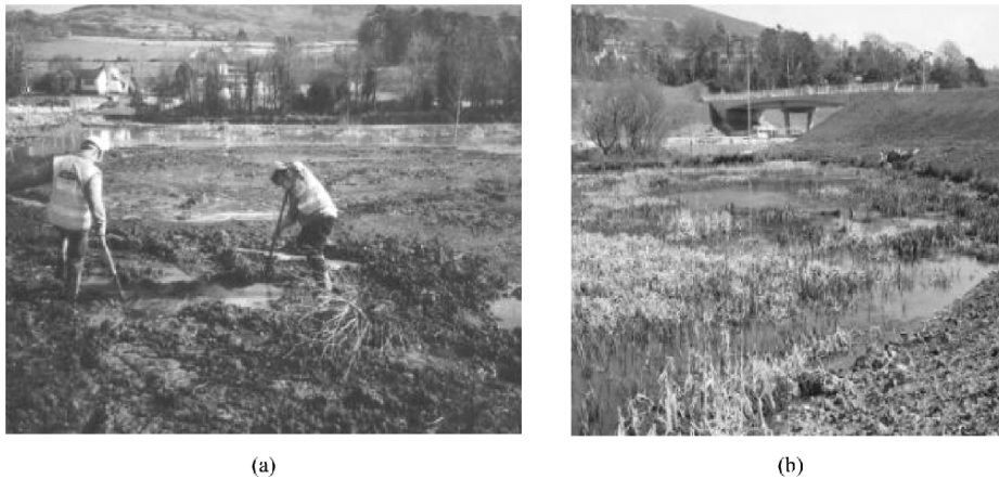
Figure 5. Translocation of marsh soils at Kilmacanogue, Co. Wicklow as part of the N11 Road scheme: (a) Before; (photograph by Richard Nairn, NATURA) (b) After (from Cullinane et al. 2003)
