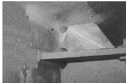
Photo 2. Fatigue cracks of steel girders
