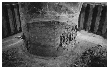
Photo 4. Hidden seismic damage of column
