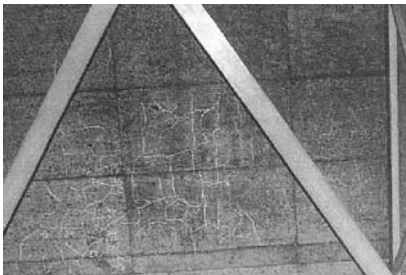
Photo 2. Deterioration of slab panels
