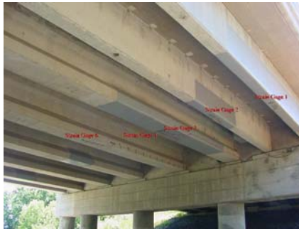
Figure 1 Instrumentation of precast prestressed girders
