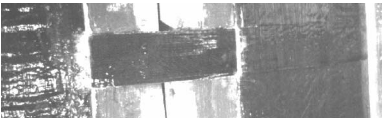
Figure 9. Crack forming in upper half of restrainer
