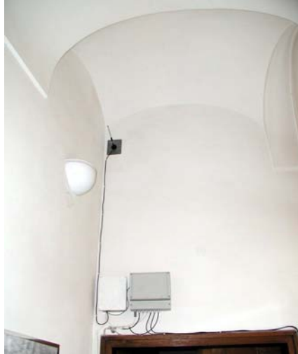
Figure 3. Data logger with transmitter in the New Town Hall in Prague.
