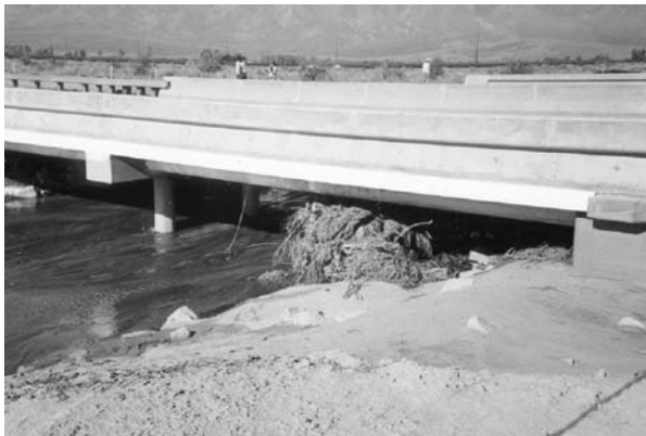
Figure 2. Floating Debris in the Form of a Tree Trunk and Roots
