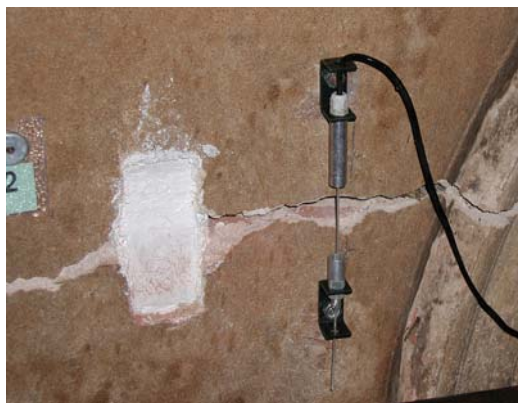
Figure 1. Traditional monitoring elements – geodetic target, gypsum strip, LVDT sensor – used for monitoring of Veltrusy Castle severely damaged by flood..
