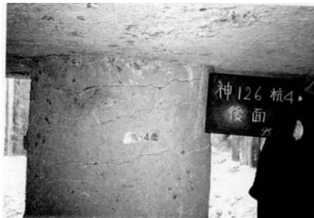
Photo 7. Typical pile damage
