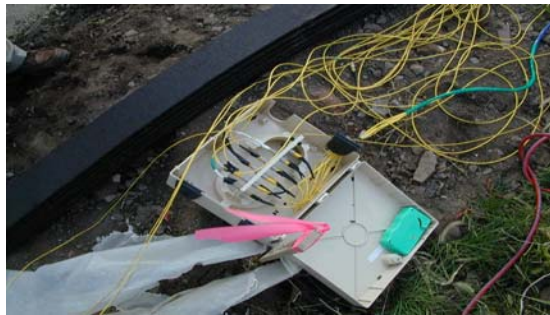
Figure 4 Temporary routing of the lead outs from the bridge deck to the junction box
