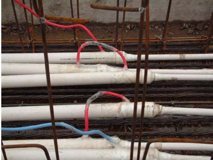
Figure 9. Photograph of connection of voltaic wires
