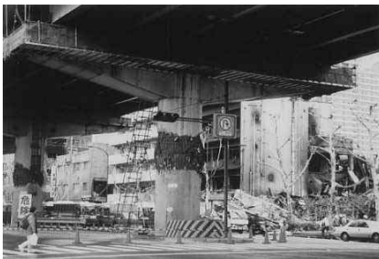
Photo 3. Seismically damaged bridge
