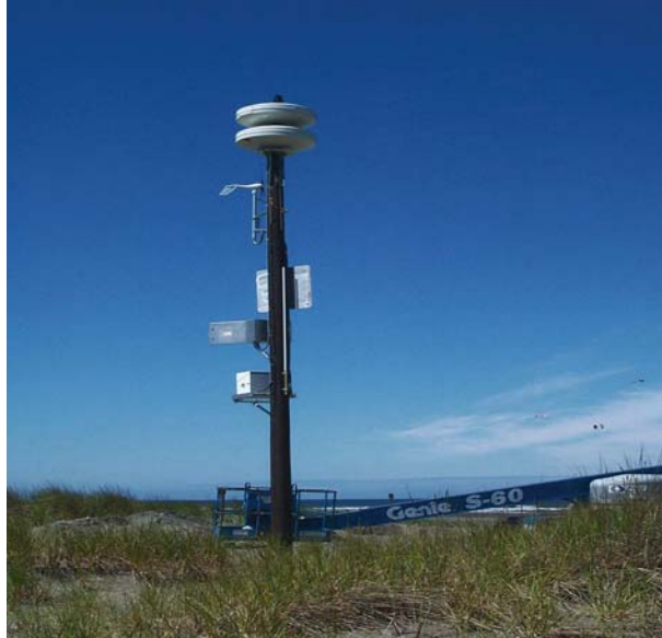
Figure 4. AHAB Radio prototype installed at Ocean Shores, Washington on 2 July 2003.
