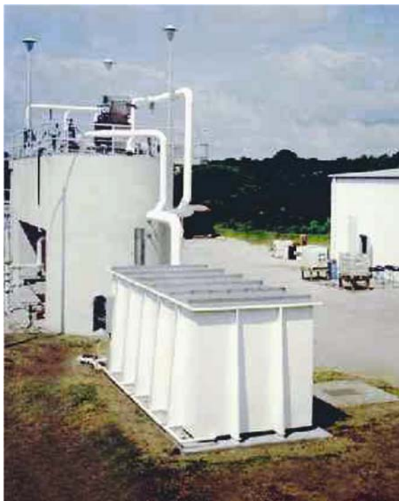
Figure 6. Picture of an actual biofilter. The in-vessel system treats H_2S and other odours at a wastewater treatment facility. The EBRT is 20 s. (Courtesy of Biorem Technologies, Inc.)
