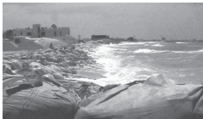
Figure 8: Deteriorating sandbags in Dubai, visual problems for local authorities (Weerakoon et al., 2003)
