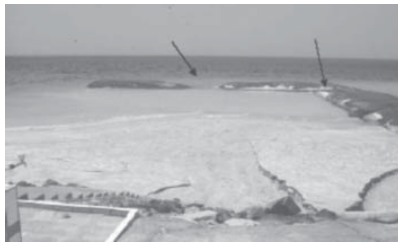
Figure 12: Slumping of a Geotube after a small storm in Dubai (Weerakoon et al., 2003)
