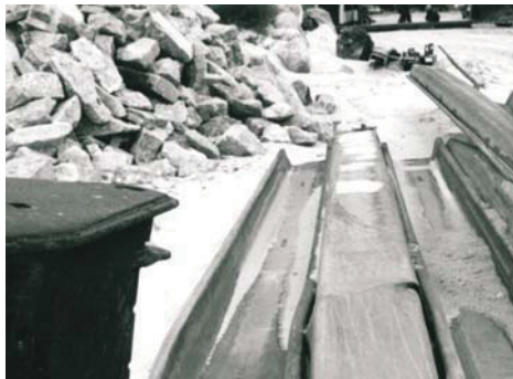
Figure 8: Damaged sheet piles
