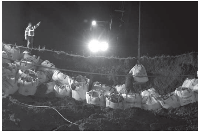
Figure 7: Emergency works at a dike breach in the Julianakanaal in the Netherlands, January 2004 (photo Michiel Wijnbergh/Hollandse Hoogte)
