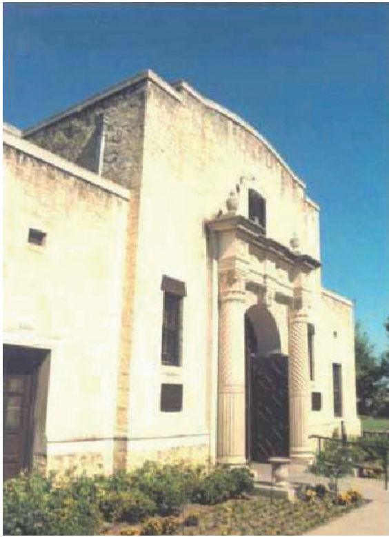
Fig. 22. Microbial adhesion and consequent deterioration only occurred at the top (dark) part of the building. The lower, protected portion was free of bacteria and deterioration.
