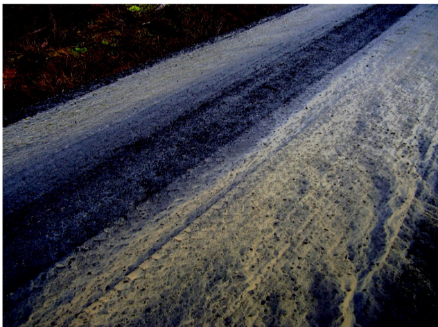
Fig. 3 Erosion from surface material during hauling
