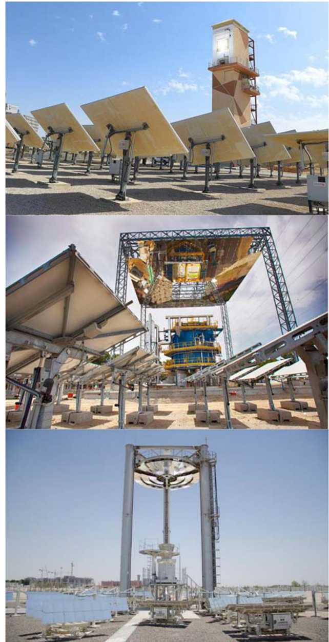
Fig. 1 Representative CSP-TES demonstrations, from top: KSA Red Sand Falling Particle Receiver/ TES Riyadh, Saudi Arabia [83••]; STEM CSP Fluidized Bed Receiver/Sand TES, San Filippo del Mela, Sicily, Italy [95]; Masdar-MIT CSPonD Volumetric Salt Receiver/ TES, Abu Dhabi, UAE [96••]
