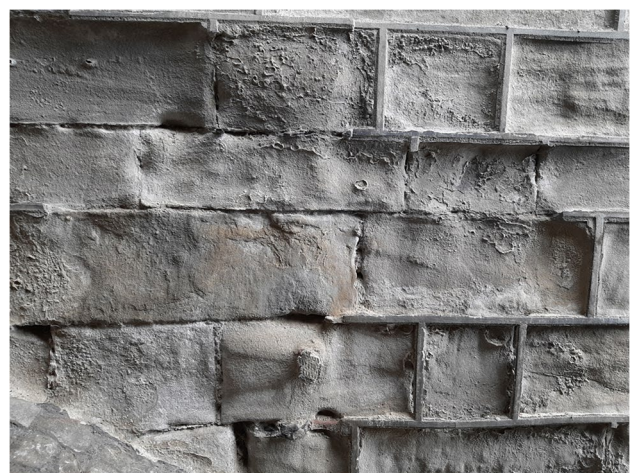
Fig. 8 Example of a reintegration of a repointing mortar. In this case, the new mortar has remained intact while the surrounding softer stone has eroded due to atmospheric agents
