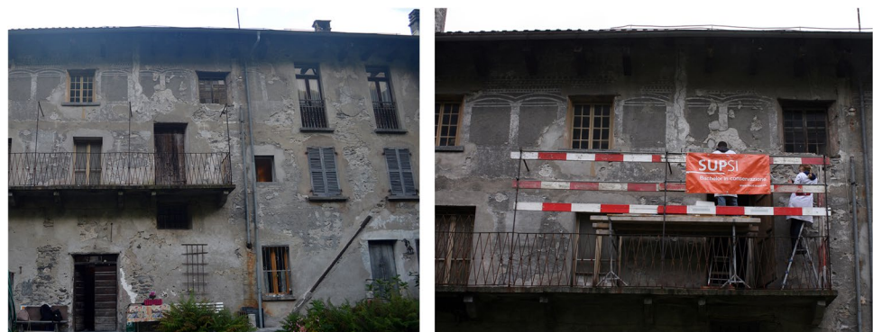
Fig. 1 Casa Zuccarelli, Ticino (CH). Examples of a decorated facade. On the left the general view of the deteriorated plaster; on the right a detail of the graffito, representing a loggia of the same façade during the conservation works
