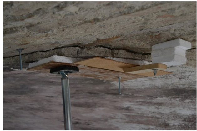
Fig. 7 Supports of a detached plaster in a vault. Supports must be ready before starting grouting, but have a fundamental role after the intervention while the grout sets
