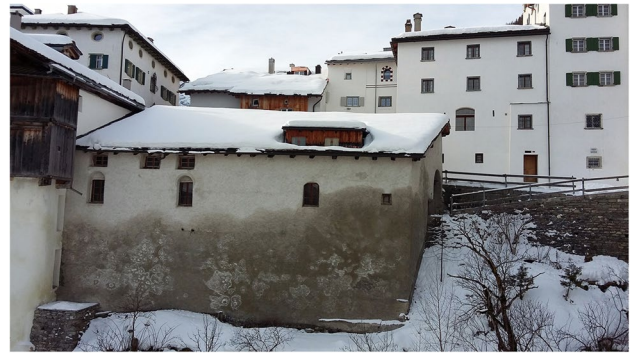
Fig. 4 Example of snow accumulation around a building, as a source of water and soluble salts. Splügen, CH
