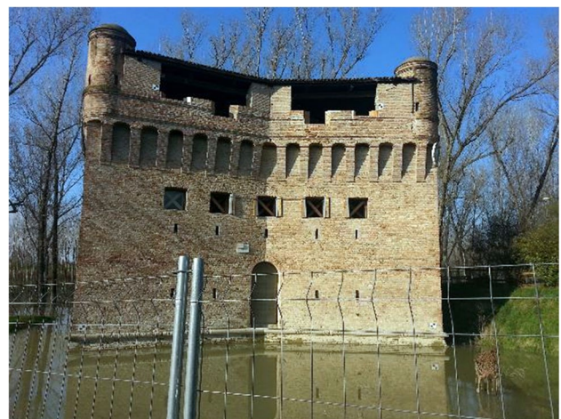
Fig. 3 The “Rocca Possente” situated in Bondeno, province of Ferrara (IT). Due to its location on the banks of the Po river, this building suffers periodic flooding and problems related to liquid water and capillary rise
