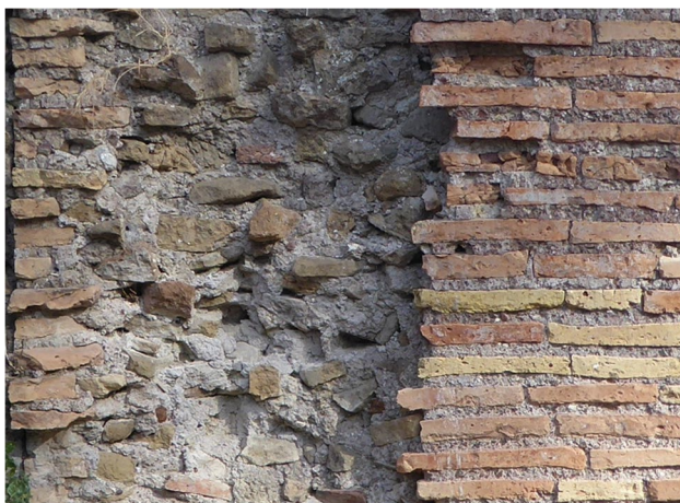
Fig. 6 Construction detail, Grandi Horrea, Ostia (Italy), late second century CE phase. Section and face of wall, from left to right: section through neatly coursed brick facing; section through roughly coursed core; neatly coursed brick facing. Photo author
