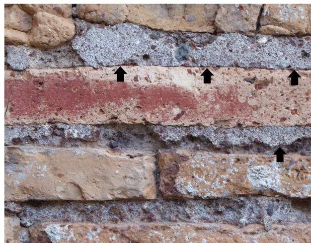
Fig. 7 Brick facing, Grandi Horrea, Ostia (Italy), late second century CE phase. Detail showing vertically struck joints (indicated by arrows); elsewhere, the surface of the mortar has deteriorated. Photo author
