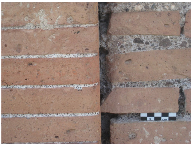
Fig. 3 Construction detail, Casa a Giardino, Ostia (Italy), built in the 120 s CE. On the right, part of wall showing standard brick facing, with mortar having a pozzolan aggregate which would go through a digitus sieve; on the left, the adjacent decorative pilaster, an integral part of the same structure, with very narrow joints requiring the pozzolan to be put through a fine sieve. Photo courtesy S. Camporeale
