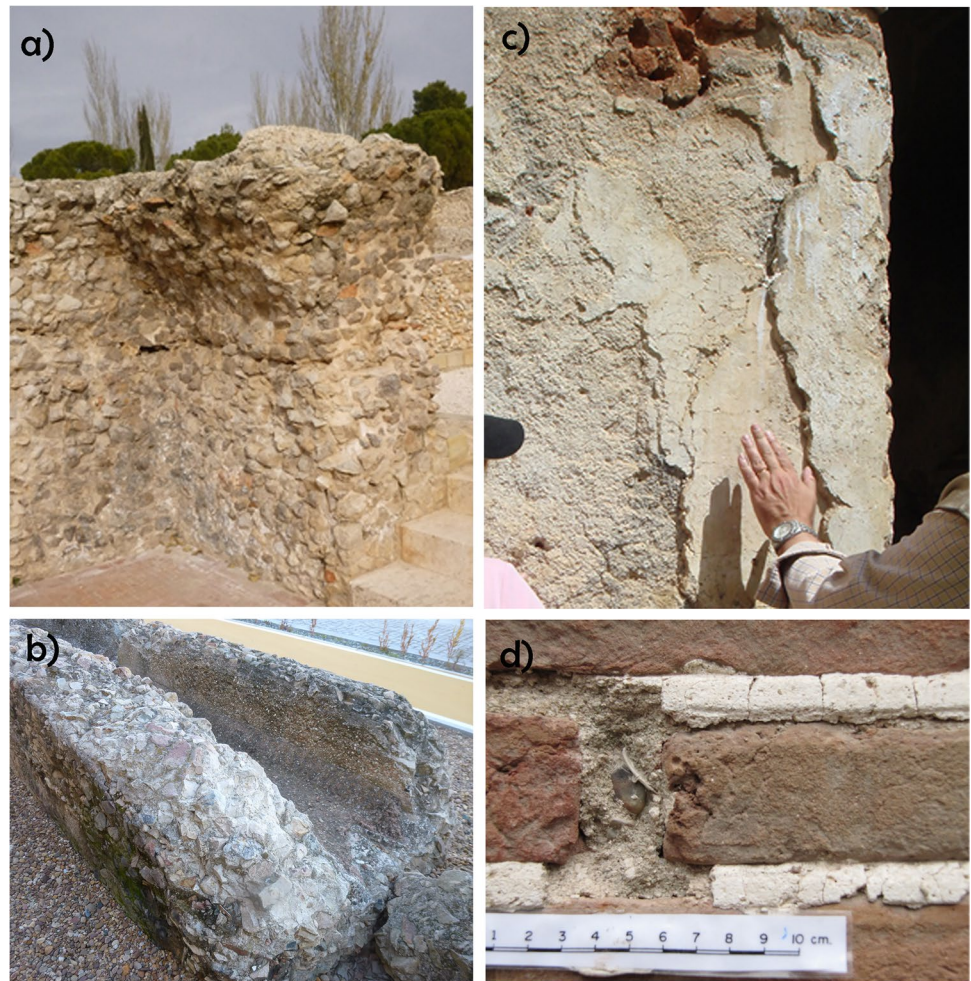
Fig. 1 Examples of aerial lime mortars/plasters in ancient and historic buildings in Spain. a Wall built with mortar and limestone pebbles (> 10-cm size) in the Roman city of Complutum, Madrid. b Part of a channel from the San Lázaro Roman aqueduct, Mérida; the base was built with aerial mortar and limestone pebbles, with several layers of aerial and hydraulic rendering mortars. c Various layers of rendering mortars applied on a wall in the Monastery of Santa María la Real in Pelayos de la Presa, Madrid, built in the seventeenth century. d Detail of bedding mortar in brick masonry at the Cistercian monastery of San Bernardo in Alcalá de Henares, Madrid, built between the seventeenth and eighteenth centuries
